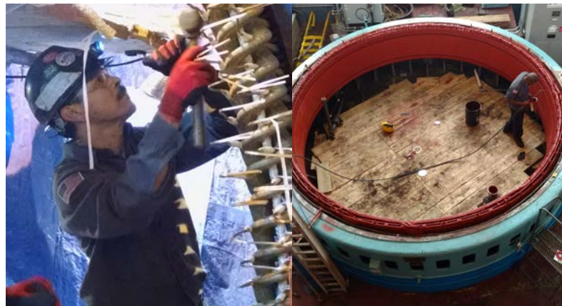
Disassembly and unstacking of thousands of laminated steel sheets to create a new stator core. Tolerance requirements were several thousandths of an inch on the bore ID.
